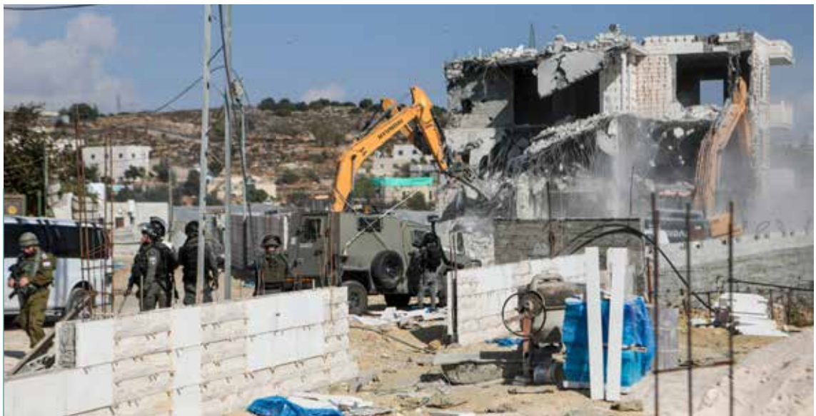
Israeli bulldozers destroy a Palestinian 3-storey building in Hebron, the West Bank, on 31 October 2022.
