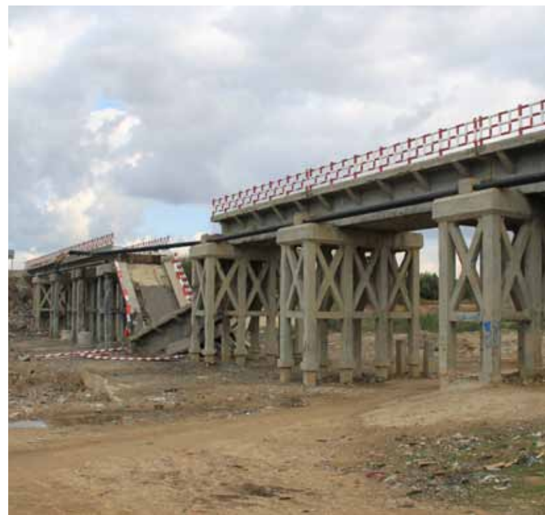
v Gaza Valley Bridge which was bombed by Israeli warplanes
