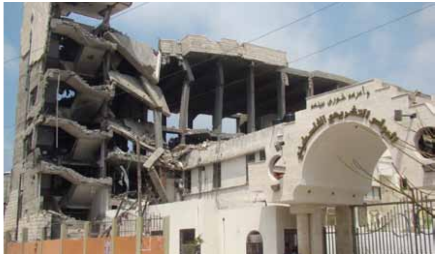
The building of the Palestinian Legislative Council, which was bombed by Israeli warplanes on 31 December 2008.
