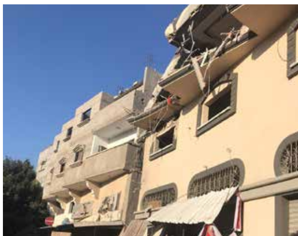
Bahaa Abulatta's house that was targeted by IOF in al-Shuja'yia neighbourhood, Gaza
