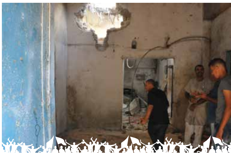
Khammash Family House Targeted and Destroyed in Deir al-Balah
